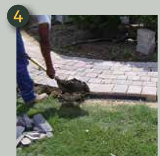
4 Backfill with soil and sod flush against the edging of the sidewall.
