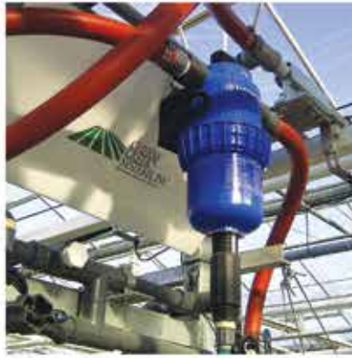
20 GPM Mounted (Cherry Creek Systems)
