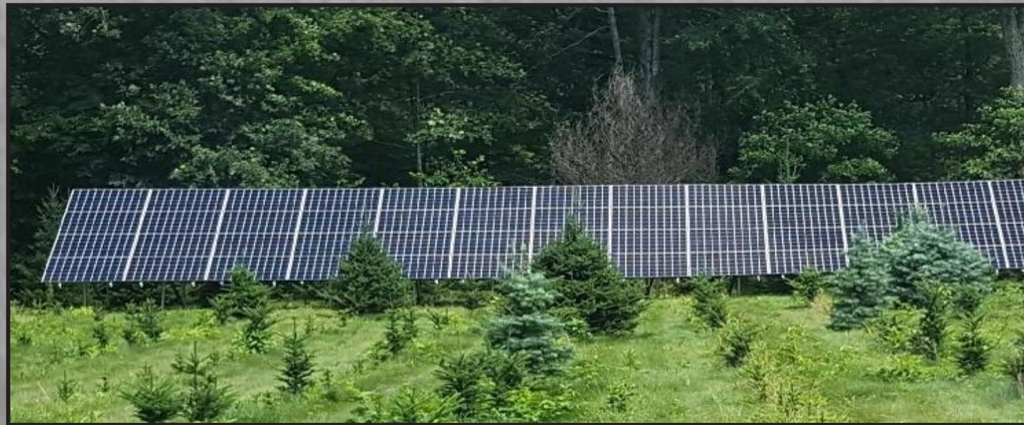
We installed a ground mounted Solar Array 18.56kW(AC) System that was turned on October, 2018.
