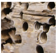
CARPENTER BEE DAMAGE
